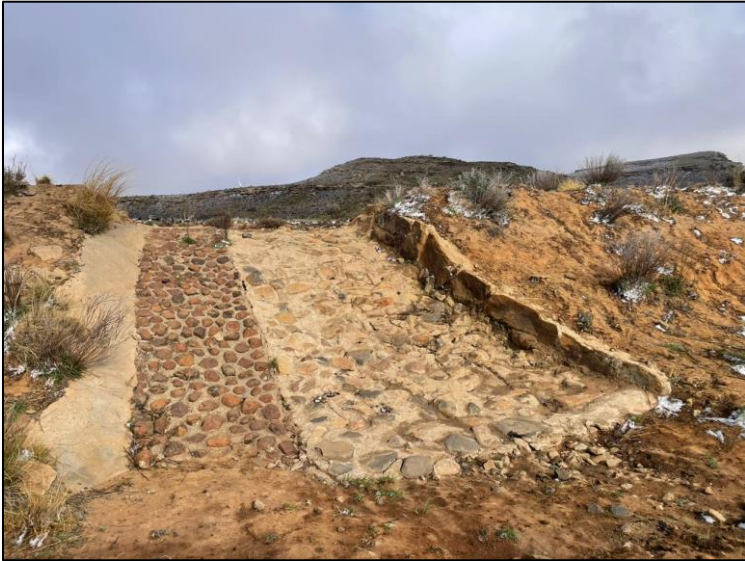
3. Stormwater infrastructure along an embankment adjacent to Road 4
