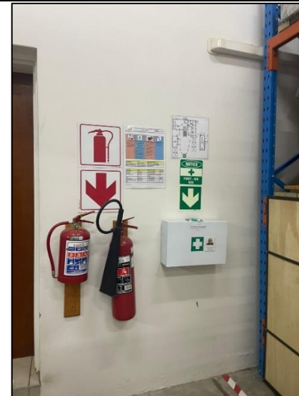
10. Health and safety signage and equipment
