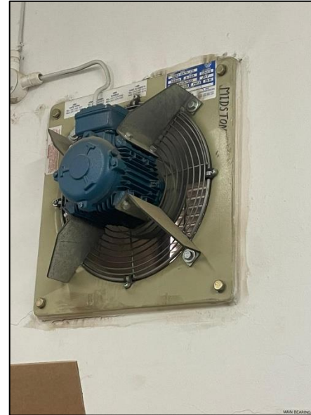
8. Chemical store fitted with extraction
